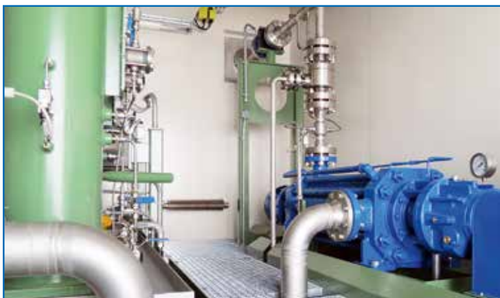
■ Apollo high-pressure injector pump skid with horizontal multistage pump
