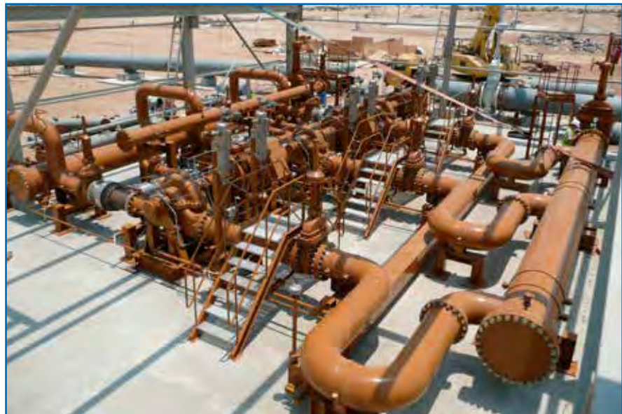
■ Booster Station for unloading of Tankers
