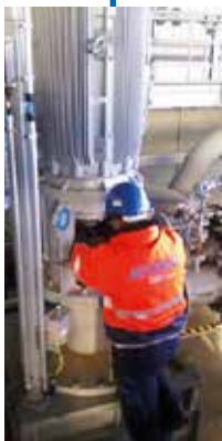
COMMISSIONING / COMPLETE ASSEMBLY ON SITE
